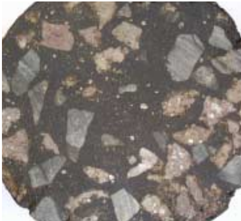
Figure 8 HRA sample containing unsound basalt aggregate that is failing due to repetitive soaking and drying
