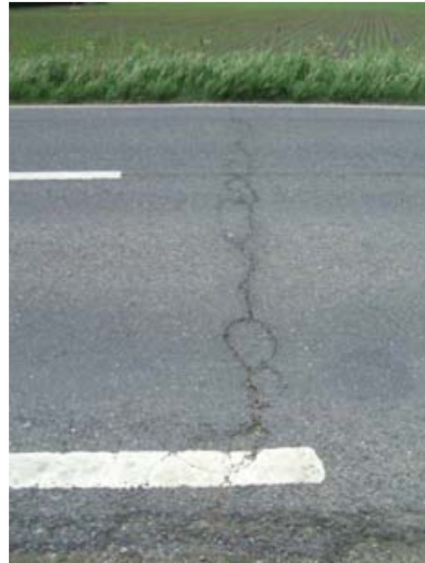
Condition 18 years later (May 2011)
