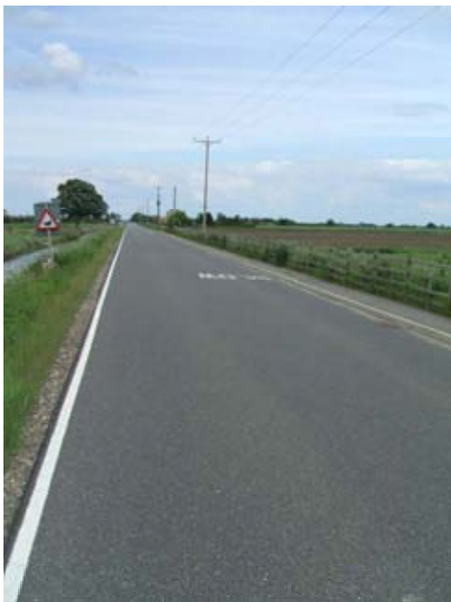
Condition after 4 years (June 2008)
