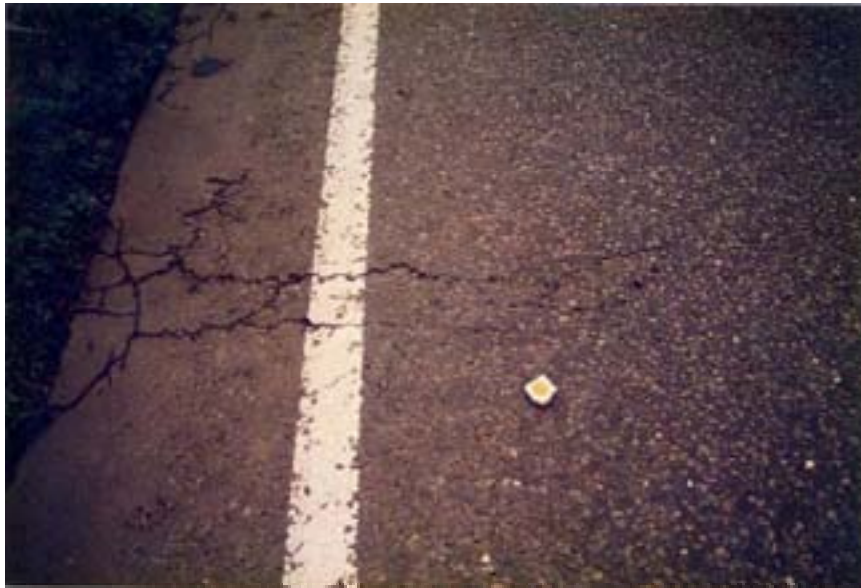
Transverse/Reflective Cracking associated with Concrete Edge Beam
