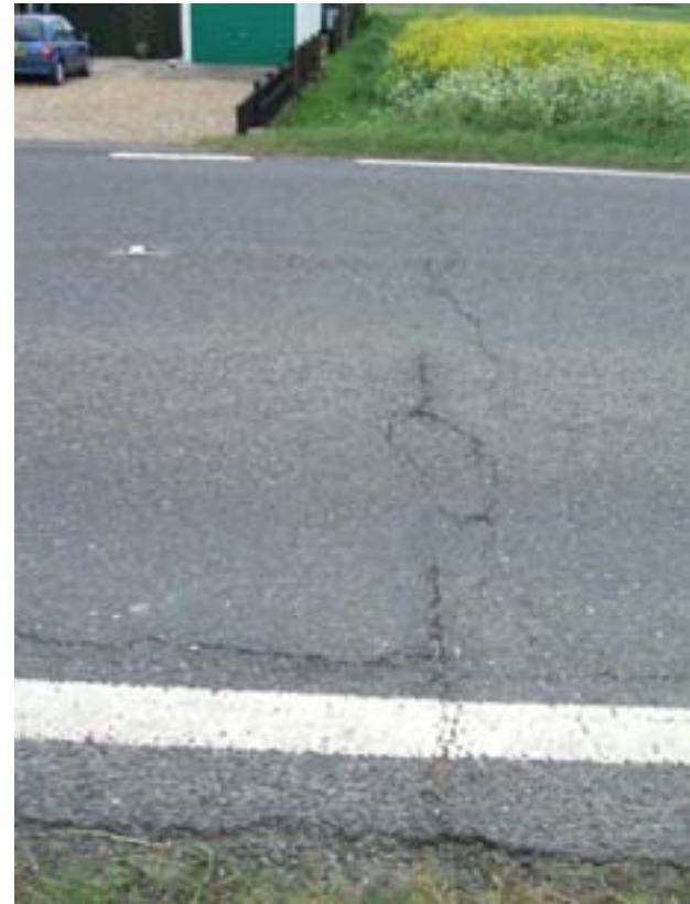
Condition 18 years later (May 2011)
